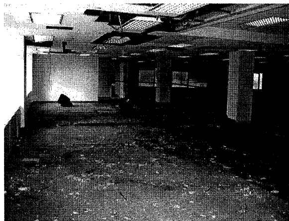
Figure 10: Floor 23 water damage
