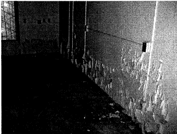
Figure 15: Floor 1 water damage
