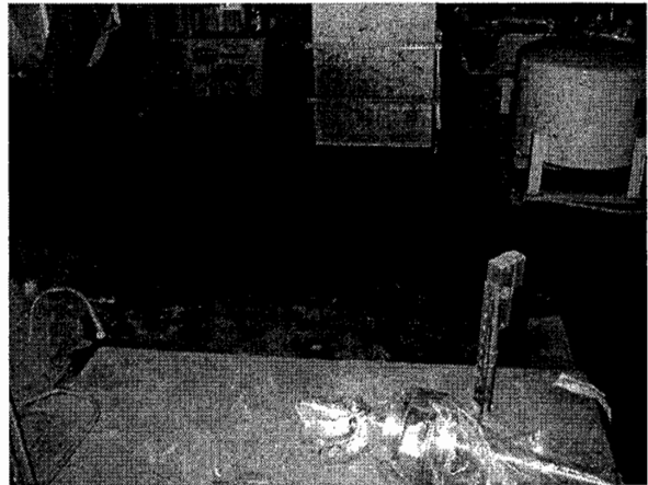
Figure 2 : Floor 40 water damage and mold.
