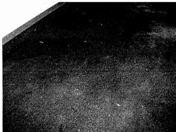
Figure 5: Floor 27 carpet water damage
