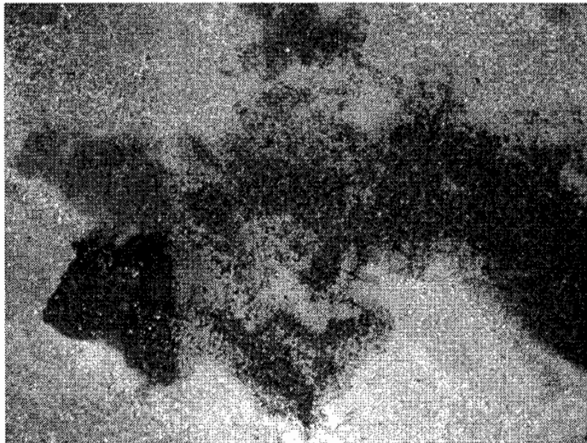
Figure 1: Floor 41 mold on flooring near pipe leak.
