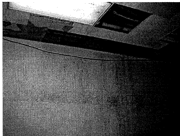
Figure 11: Floor 22 water damage
