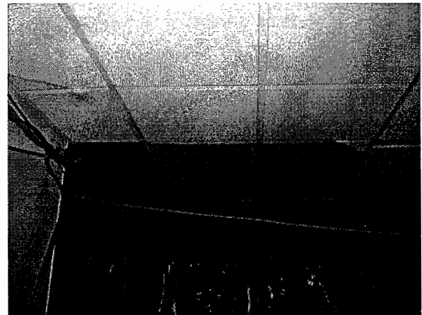
Figure 4: Floor 39 water damage.
