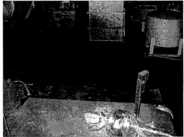
Figure 2 : Floor 40 water damage and mold.
