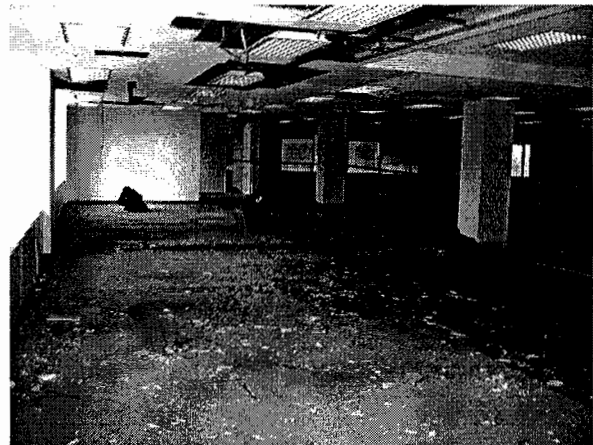
Figure 10: Floor 23 water damage
